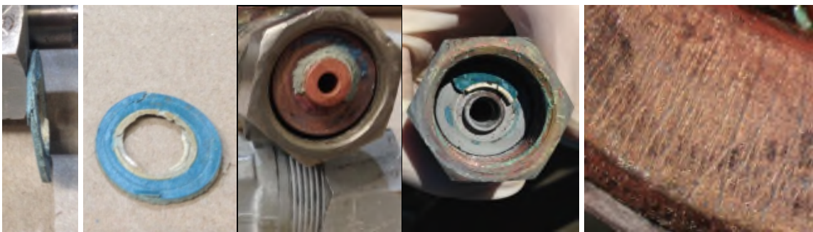
Figure 3: 1. Unevenly compressed gasket, 2. Torn gasket, 3. Gasket stuck to sealing face, 4. Broken gasket, 5. Scratches on valve sealing face
